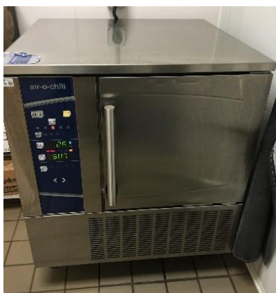
Exterior of Blast Chiller
