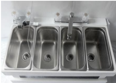
Fixed handwash as part of 3-compartment
