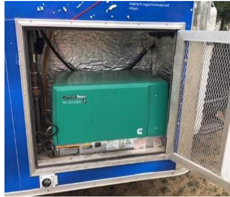
Generator installed in exterior compartment of unit
