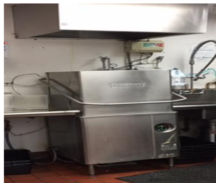
Type II hood over heat/moisture producing dishmachine
